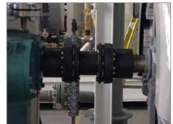
Rexnord® Thomas Disc Coupling hub mounted to water pump from motor using a TLK600 external locking device
